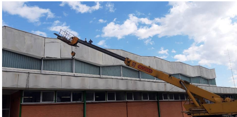
Page 4 The hoist that raises the photovoltaic on the roof of the sports hall
